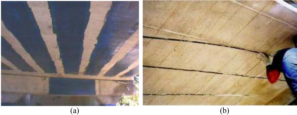
Fig. 6.1. FRP applications for deck slab (courtesy of Tarek Alkhrdaji): (a) externally bonded FRP sheets; (b) near-surface mounted FRP strips
