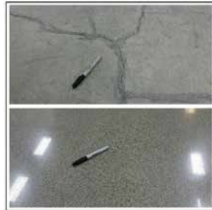
Fig. 1: A properly repaired crack will be difficult to see after the floor is polished
