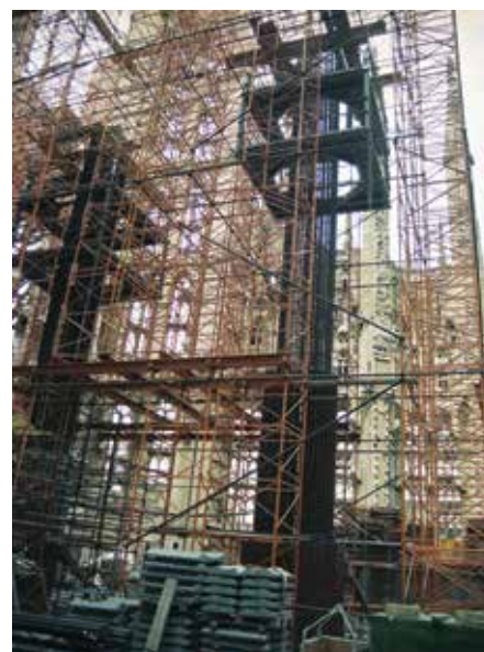
Fig. 5: Construction of the interior columns was completed inside the existing façades between 1991 and 2003 (© Fundació Junta Constructora del Temple de la Sagrada Família)
