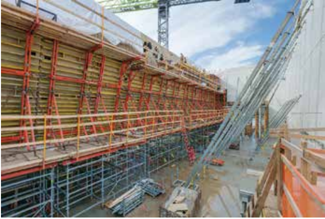
Fig. 11: A view of the interior shoring and formwork required to construct the curved wall of the River Pavilion
