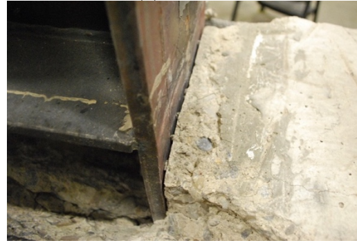
(d) Gap opening between flange and wall
