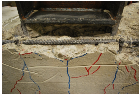
(c) Damage penetration
