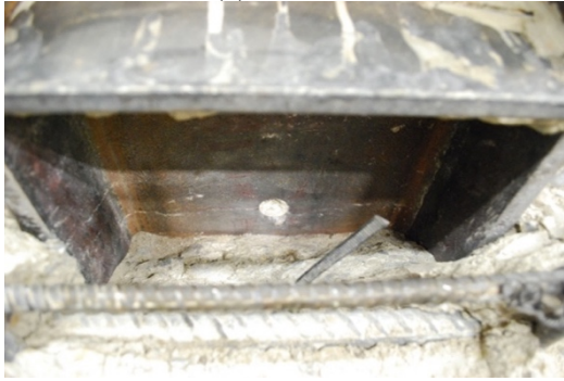
(c) Damage penetration
