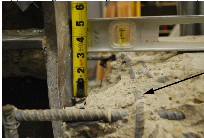
(e) Damage around flange
