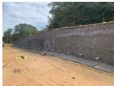
Soil nails and wired mesh installed during the early stages of a soil nail wall
