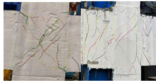
(a) Middle joint in specimen F
