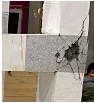
(a) Damage to the exterior joint of specimen F
