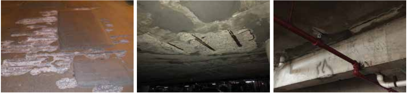
Fig. 4: Examples of corrosion-related distress adjacent to repair areas
