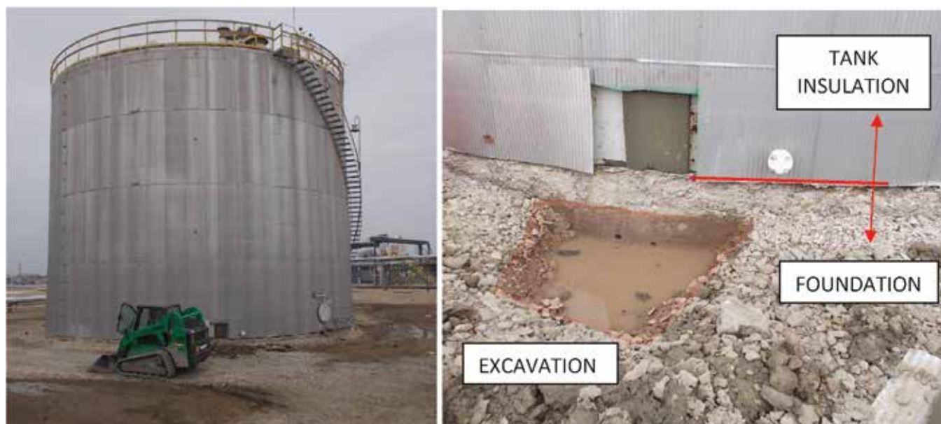
Fig. 2: Overall and close-up view of deteriorated storage tank foundation (Fig. 5.1 in Reference 3)
