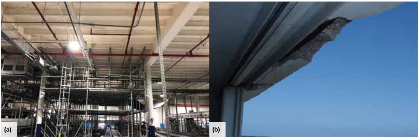
Fig. 2: Examples of potentially dangerous structural conditions: (a) overhead spalling hazard; and (b) shoring of structural concrete components with deficiencies
