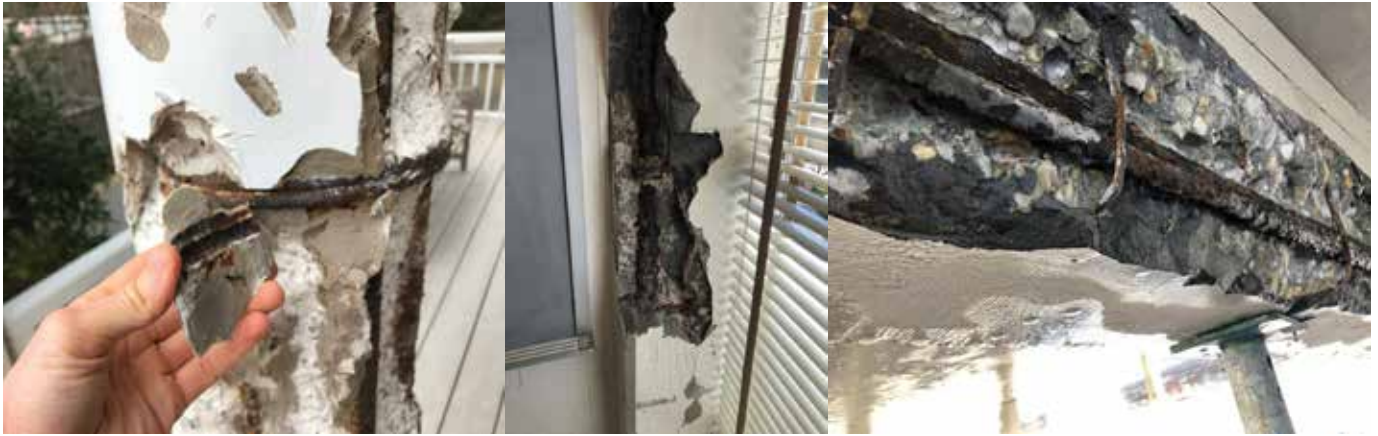
Fig. 1: Examples of failed concrete repairs
