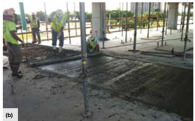
Fig. 1: Pour strips are gaps in floor structures designed to minimize restraint of early stage volume changes of concrete: (a) backshoring and changes in elevation create logistical and scheduling issues; and (b) delayed concrete placements result in high unit costs
