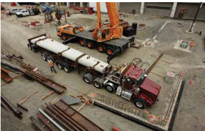
Walls weighed from 45 to 93.5 tons (41 to 85 tonnes) and were delivered using special transports
