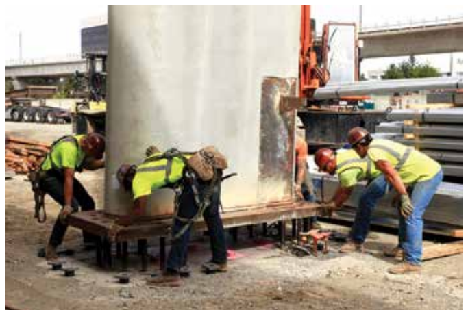
Wall units were handled using rigging inserts placed on the manually finished side, and they were anchored to foundations using cast-in-place anchor rods
