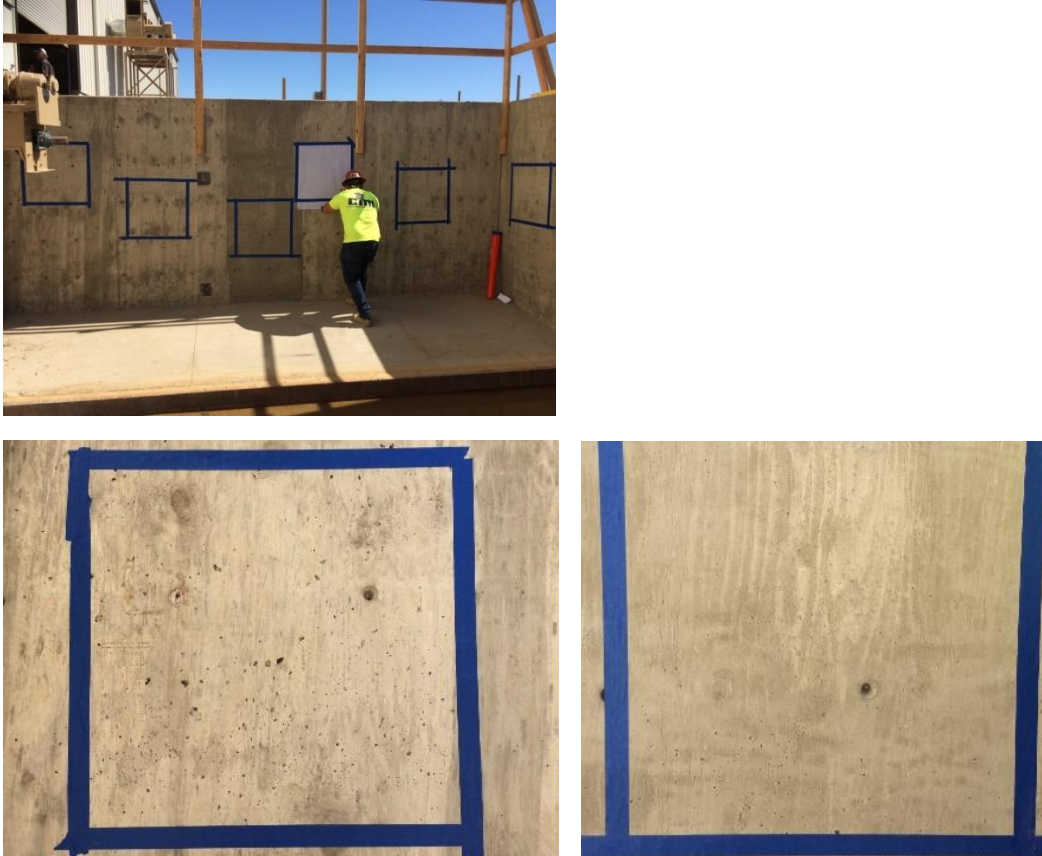
Fig. 6.16 Wall at a warehouse dock measured for SVR by University of California-Chico student researchers
