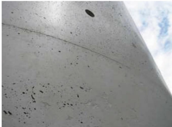
(a) General view of formed surface with high ratio of surface voids and imperfections
