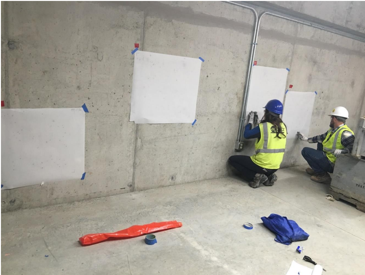
Fig. 6.10 Parking garage and office complex walls measured for SVR by MTSU student researchers
