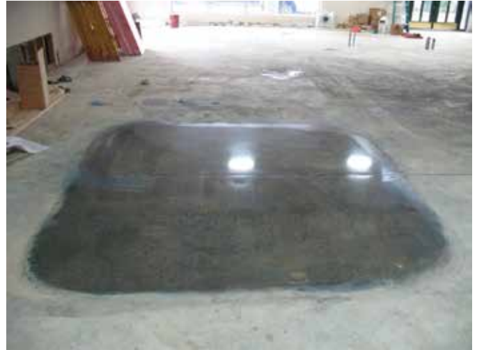
Fig. 10: An example of a ground mockup section where a superficial weak area was removed, exposing dense concrete layer below
