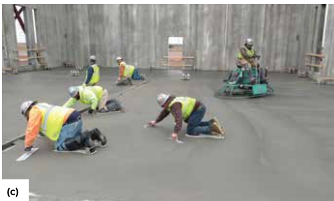
Fig. 7: Concrete slab surface: (a) after removal of rainwater, with a close-up showing the sandy appearance of the surface; (b) after the first pass of a ride-on trowel; and (c) during final finishing
