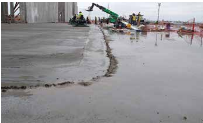
Fig. 8: Finishers used dry cement to create a dam outside of the fresh concrete placement and prevent previously removed rainwater from flowing back onto the working area. The dry cement was removed shortly after final finishing
