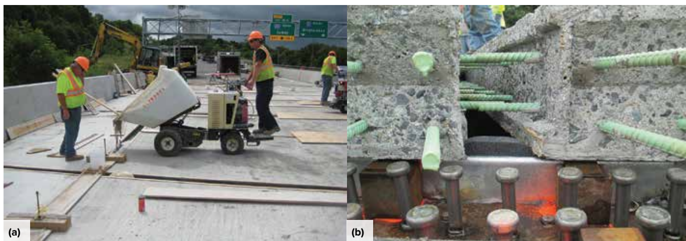
I-81, Syracuse, NY: (a) field-casting of UHPC on an interstate bridge construction project; and (b) UHPC connection between precast deck panels and between panels and the girder (photos courtesy of Ben Graybeal)
