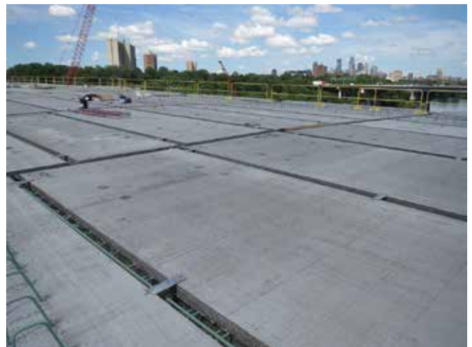
Precast deck panel placement prior to UHPC connection casting, Franklin Avenue Bridge, MN (photo courtesy of Ben Graybeal)
