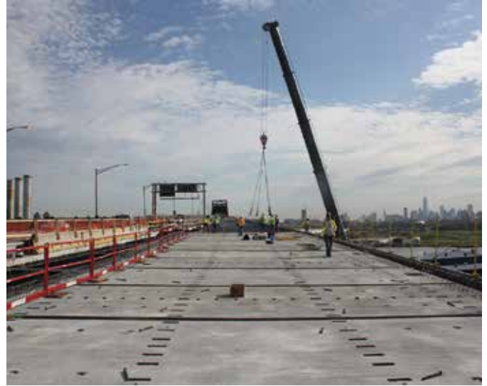
Precast deck panel placement prior to UHPC connection casting, Pulaski Skyway, NJ (photo courtesy of Ben Graybeal)
