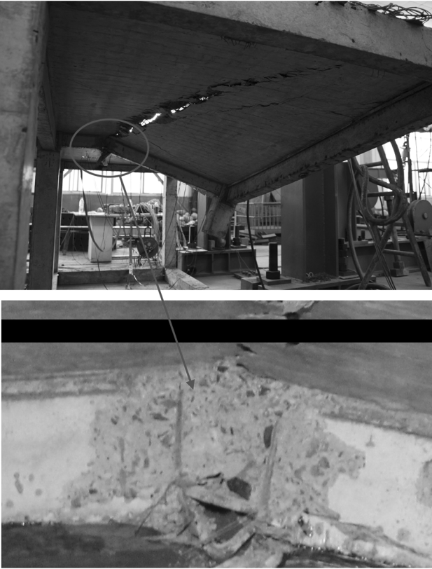
Fig. 9 Failure of frame beam and slabs in short axis direction at collapse limit state.
