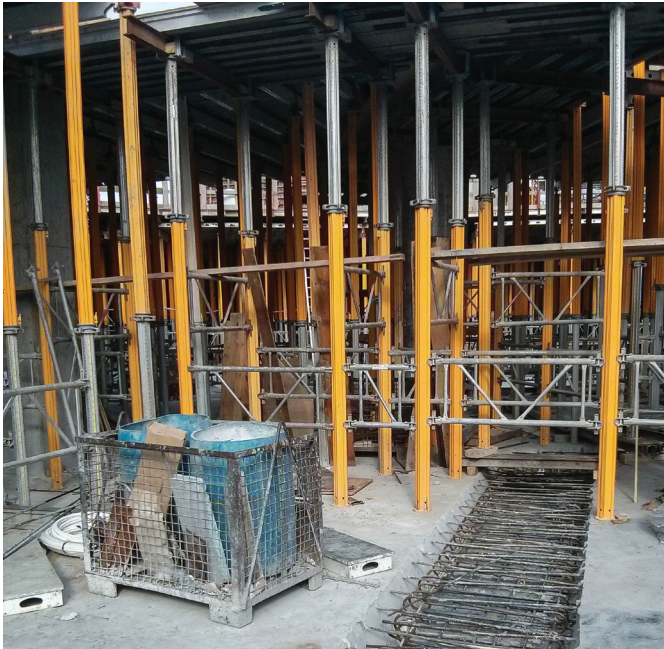
Fig. 8: Shoring for the next floor built directly above an open closure strip (photo courtesy of A. Brault)
