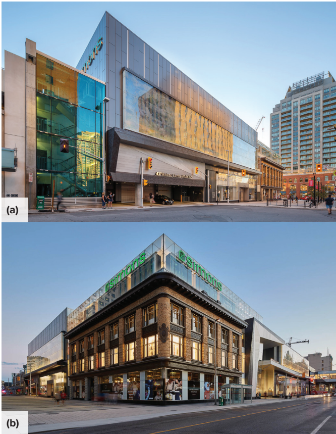
Fig. 2: The Rideau Centre Expansion construction project, Ottawa, ON, Canada, served as field monitoring site (photos courtesy of doublespace photography)
