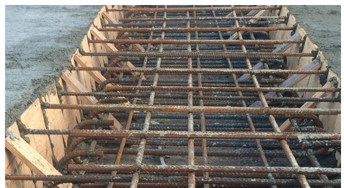
Fig. 1: A 1 m (3.28 ft) wide closure strip before concrete placement (photo courtesy of A. Brault)
