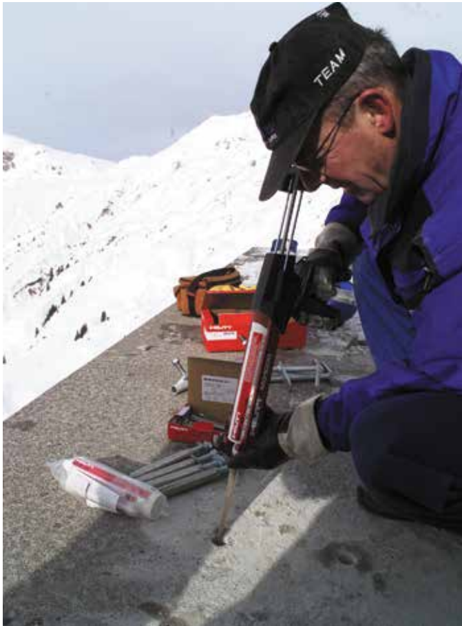
Fig. 2: Injecting adhesive using a hand-operated injection tool—the adhesive is mixed in the static mixer attached to the end of the tool. The MPIO must be consulted to ensure that the adhesive is appropriate for the ambient conditions
