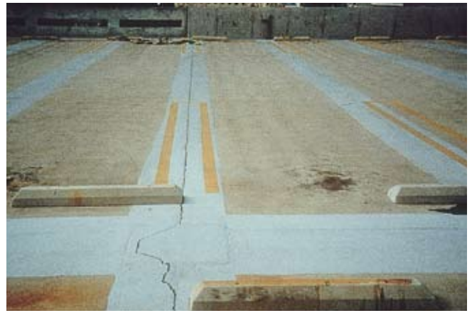
Fig. 2. Concentrated cracks along column lines.
