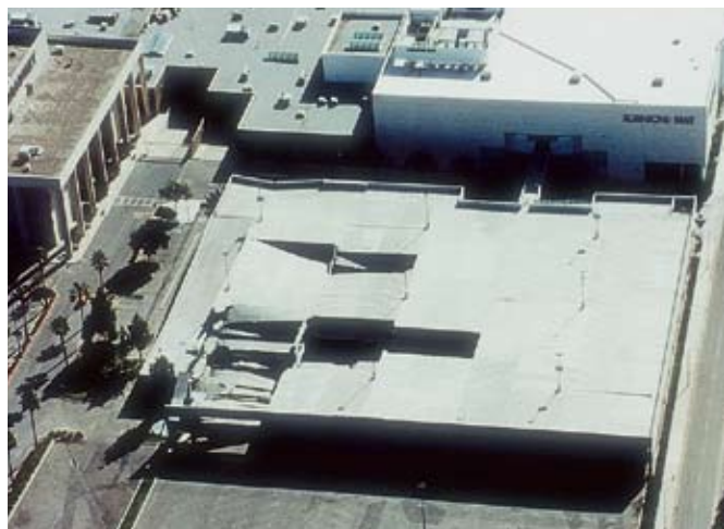
Fig. 3. Partial collapse of parking structure in Northridge, California.
