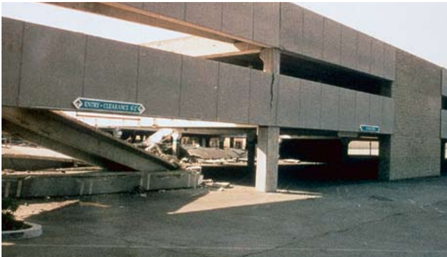
Fig. 5. Structural walls remained uncracked while precast concrete elements collapsed in parking structure in Northridge, California.
