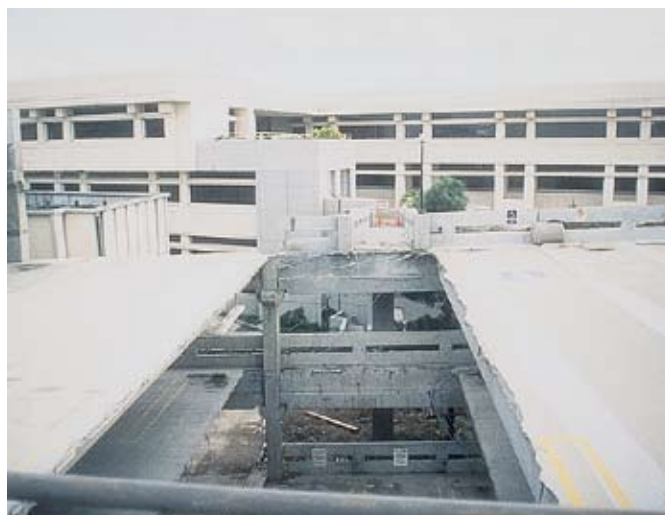
Fig. 4. Partial collapse of parking structure in Glendale, California.
