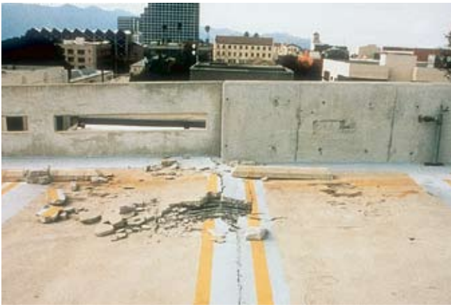
Fig. 1. Buckled chord reinforcement in diaphragm.
