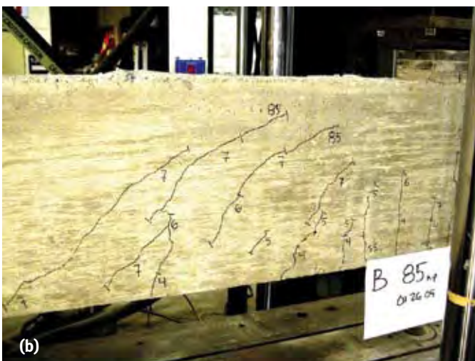
Fig. 2: Typical cracking patterns for beams tested at the University of Michigan: 4 (a) reinforced concrete beam without steel fibers; and (b) reinforced concrete beam containing steel fibers
