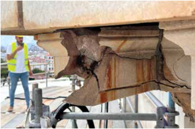
Dome's base ornamental friezes showing corrosion and cracking
