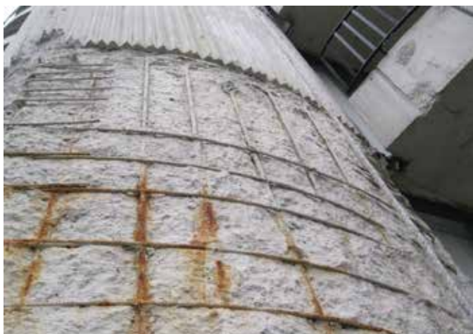
Fig. 2: Premature corrosion of reinforcing steel due to inadequate concrete cover
