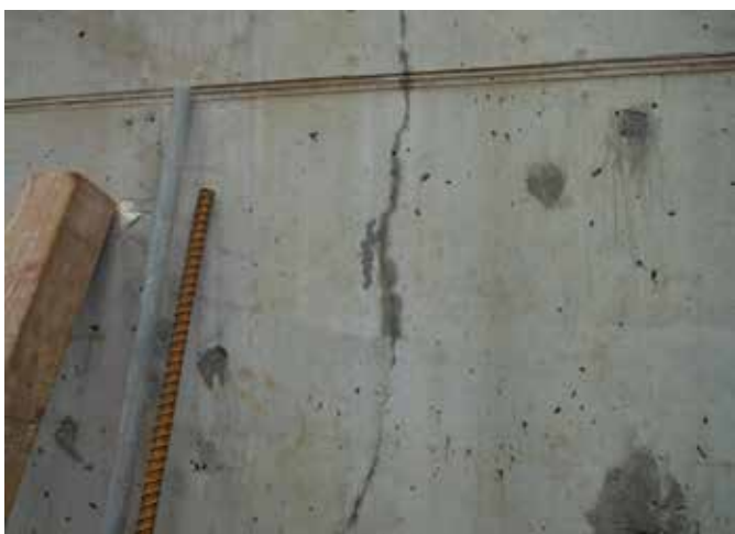
Fig. 3: Cracking in this concrete structure may have a significant impact on its durability
