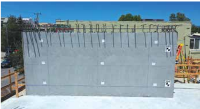
Fig. 3: Concrete wall with fine chalk lines
