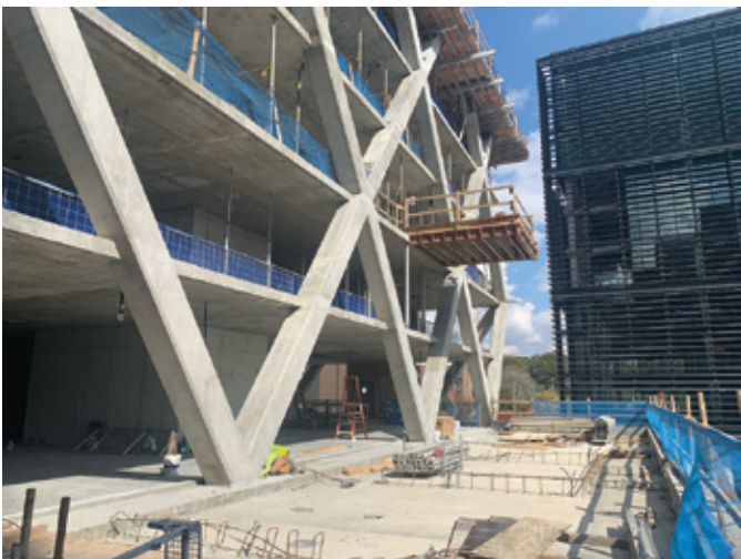
Fig. 2: View of the façade showing the columns sitting 12 in. (305 mm) proud of the slab
