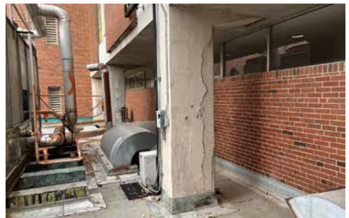
Fig. 3: Vertical cracks and concrete delamination in a column
