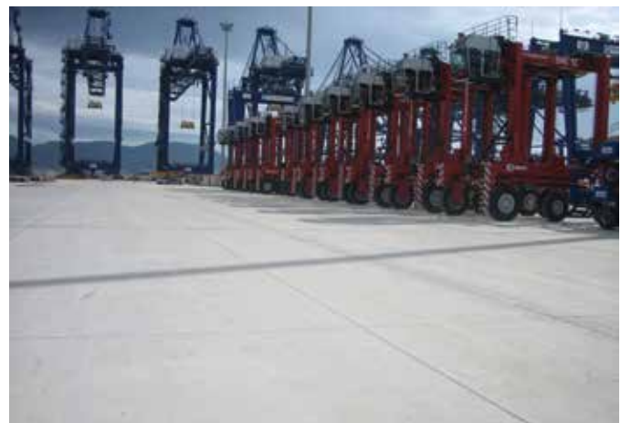
Fig. 1: Pavement with Type I steel fibers at the Maersk Container Terminal, Algeciras, Spain, constructed in late 1990s
