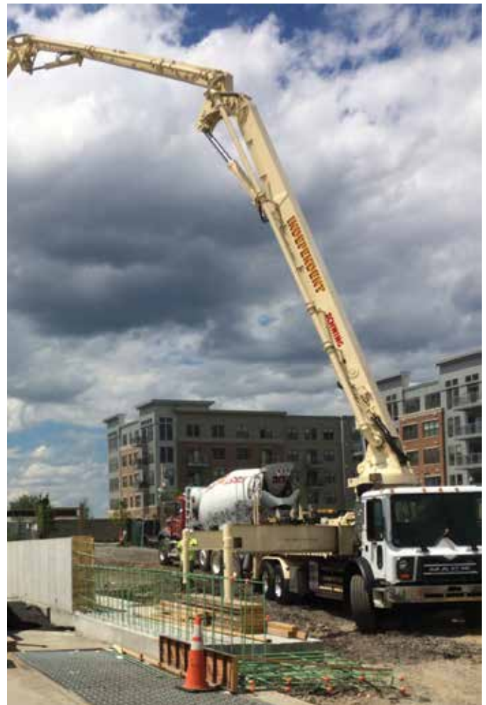
Almost all lightweight concrete used in elevated floor slabs is pumped (photo courtesy of William H. Wolfe)
