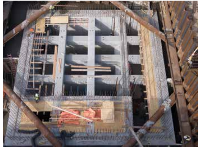
Argentine Main Pump Station
