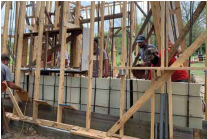
Fig. 2: Insulation was installed in the middle of wall formwork before concrete placement
