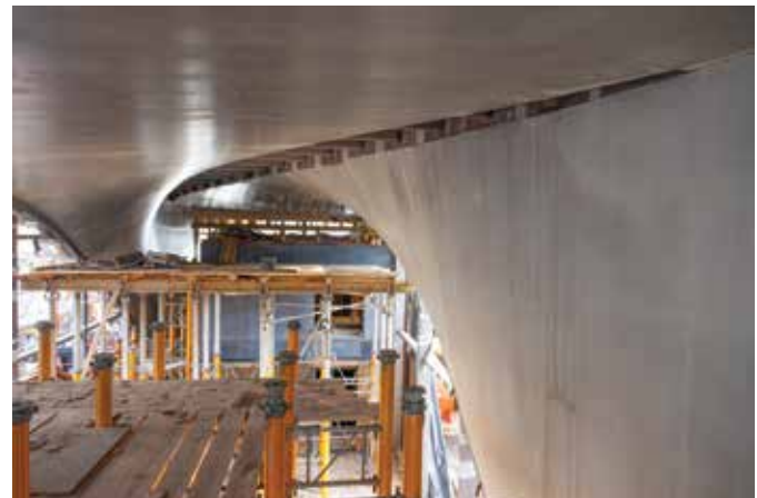
Fig. 3: The curved portion of the wall system was constructed using a factory-built form brought on site (photo courtesy of Stefan Groeschel, IMB, TU Dresden)
