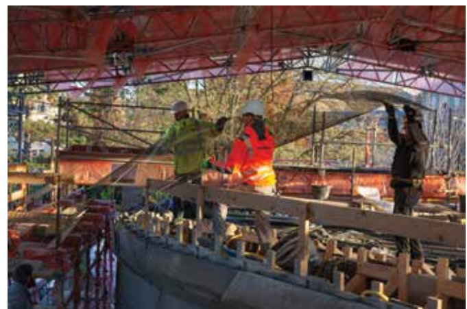
Fig. 4: Workers carrying carbon textile used for construction of carbon textile concrete elements of the structure (photo courtesy of Stefan Groeschel, IMB, TU Dresden)
