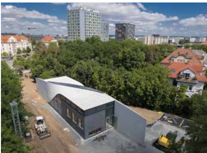
Fig. 1: The Cube during construction with a simple box design and a roof sloping into a wall (photo courtesy of Stefan Groeschel, IMB, TU Dresden)
