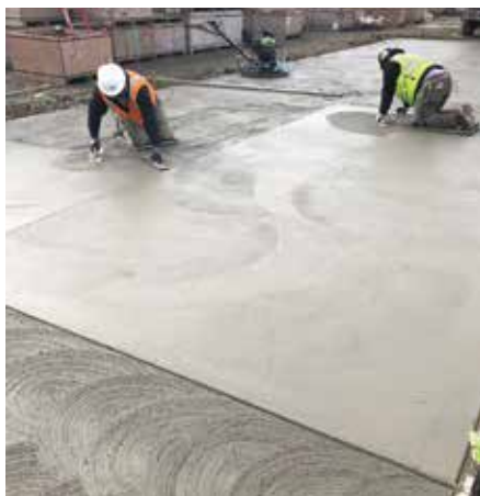
Fig. 6: For a broom finish, after panning, finishers on kneeboards used a hand float and trowel to prepare the surface for brooming. The swirl finish was placed on the panned surface
