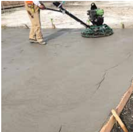
Fig. 5: After the channel float and waiting time, workers used a 36 in. (914 mm) walk-behind machine with a pan
