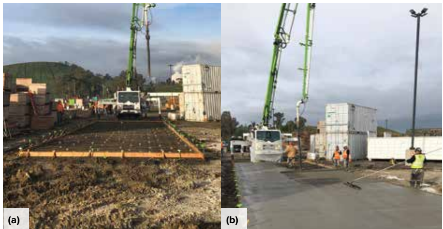
Fig. 4: Initial steps in the construction of a 20 x 80 ft (6 x 24 m), 6 in. (150 mm) thick test panel used to evaluate the effects of swirl and broom finishes on F-numbers: (a) formwork, reinforcement, pump, and crew are in place; and (b) concrete placement nearing completion. Concrete was pumped, internally vibrated, struck off using a 16 ft (5 m) long screed, and smoothed using a 6 ft (2 m) channel float
