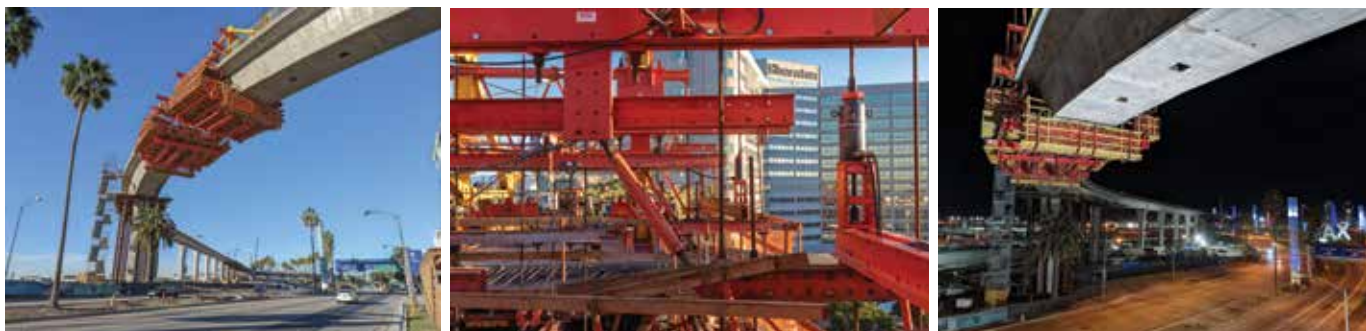
The PERI VARIOKIT system in use during construction of the Automated People Mover at LAX in Los Angeles, CA, USA (photos courtesy of Arellano Associates)
