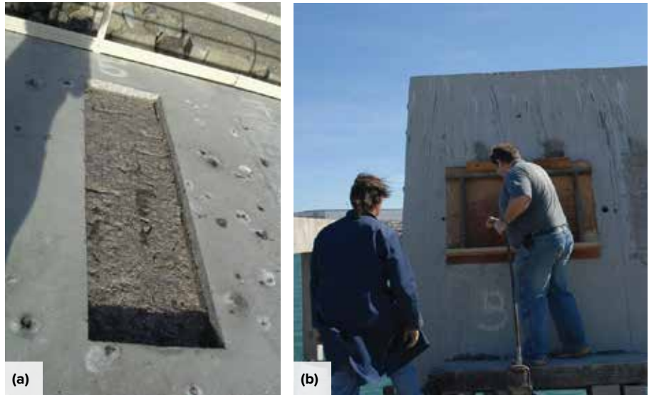
Fig. 6: Repair areas selected for field experiments at the U.S. Navy facility in Port Hueneme, CA, USA: (a) horizontal, on the pier, 73.5 x 19.5 in. (1840 x 490 mm) and 3 in. (75 mm) deep; and (b) vertical, on an existing slab installed upright next to the selected pier, 48 x 36 in. (1200 x 900 mm) and 3.5 in. (88 mm) deep 5
