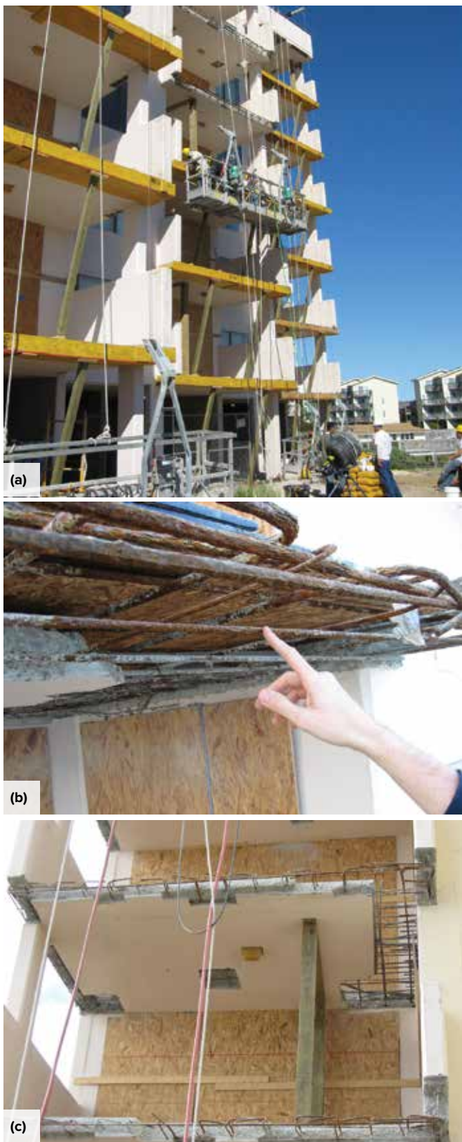
Fig. 4: Balcony repairs: (a) general construction access with visible swing stage; (b) extent of distress; and (c) one of the more severely distressed balconies requiring shoring. Note demising walls at balcony sliding glass doors
