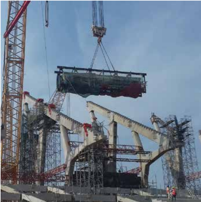
Fig. 13: A precast concrete circumferential beam is lifted into place. The beam is enclosed in a bespoke truss assembly to allow safe completion of cast-in-place connections to the radial frames
