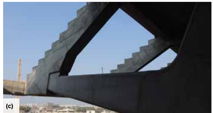
Fig. 12: The columns were produced with structural steel embedments at upper connection points: (a) embedments extending from column end; (b) corresponding pockets in bottom of PRB; and (c) a completed connection of a column end to a PRB
