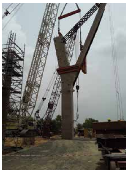
Fig. 10: A view of an HY column after erection. During rotation, the column was reinforced with a truss tie between the two arms and a strongback extending along the slender arm
