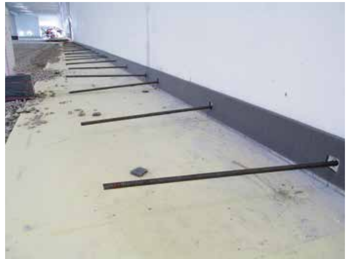
Fig. 1: Steel threaded coil rods anchored into concrete wall panels and positioned for embedment along the slab-on-ground perimeter
