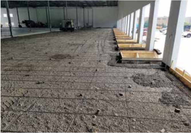
Fig. 3: Slab-on-ground steel reinforcing quantities and details redesigned to be within ACI 360R recommendations while still providing restraint for the concrete wall panels
