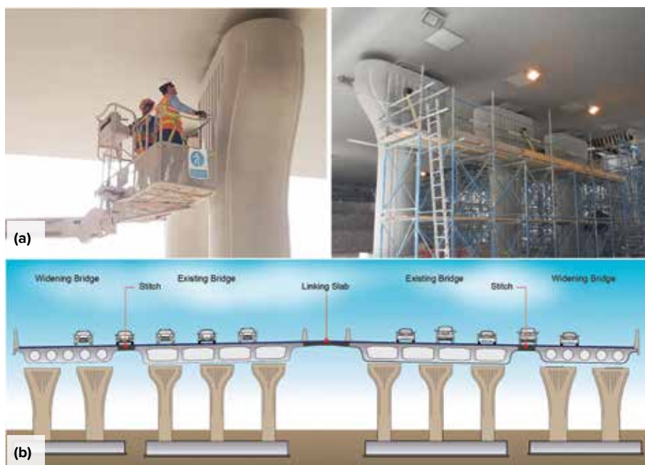
Fig. 3: Existing bridges were integrated into the project: (a) condition survey; and (b) schematic of widening scheme
