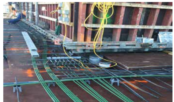
Fig. 4: Tendons routed outside of structural walls. This may be possible on short walls but is more difficult to achieve with longer walls
