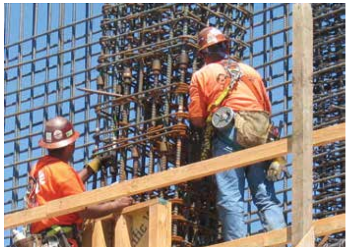
Detailing columns with mechanical couplers can help reduce congestion and improve constructability (photo courtesy of Tipping Structural Engineers)
