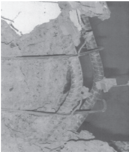
Fig. 4 Typical buckling of longitudinal bar in a spiral-reinforced column.
