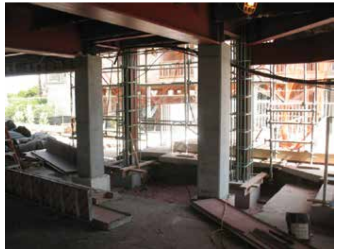
Hyperion Towers project credits: Hyperion Towers Homeowners Association, Owner; SKA Consulting Engineers, Inc., Engineer; Heard Ratzlaff Construction, Inc., Contractor; and Ready Mixed Concrete Company, Concrete Supplier
