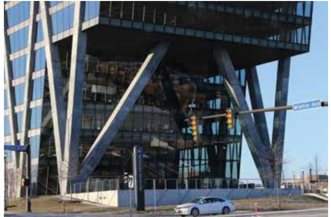
Fig. 6: The “tree columns” consist of three columns originating at a common node at the ground floor. Two branches inclined at 34 degrees from vertical support interior columns at level 6
