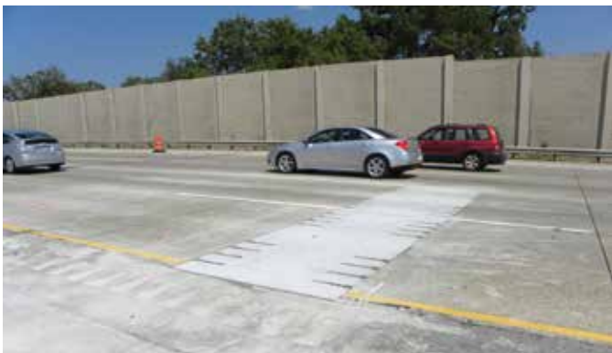
Fig. 4: A repair made using the Illinois Tollway version of a surface slot system
