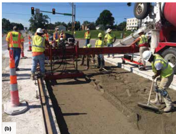
Fig. 1: Grade supported panel placement: (a) schematic; and (b) cement-treated bedding layer placement
