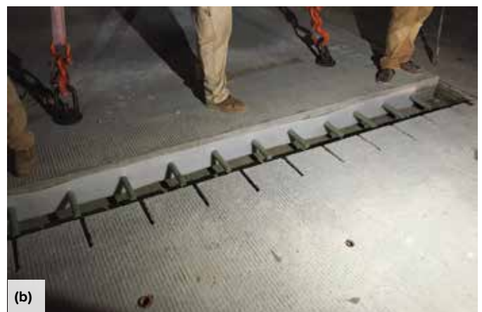
Fig. 6: California teardrop-shaped surface slot: (a) shape of slots; and (b) panel installation
