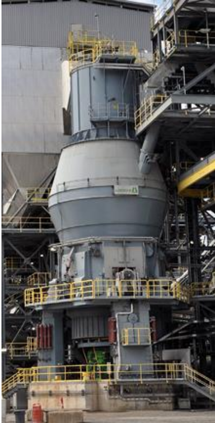
Vertical Roller Mill
