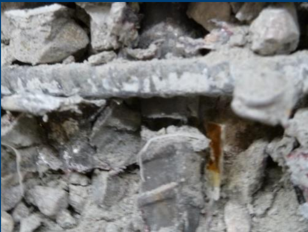
9.0% Drift Ratio (1 st Rebar Rupture)
