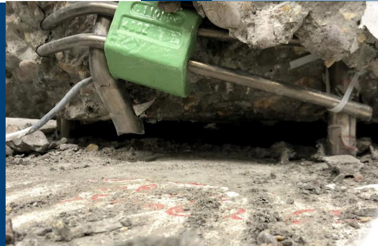
12.38% Drift Ratio (Bar Rupture)
