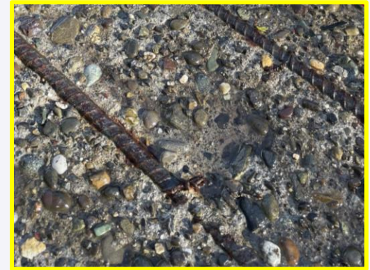
Exposed Aggregate & Rebar (ER)
