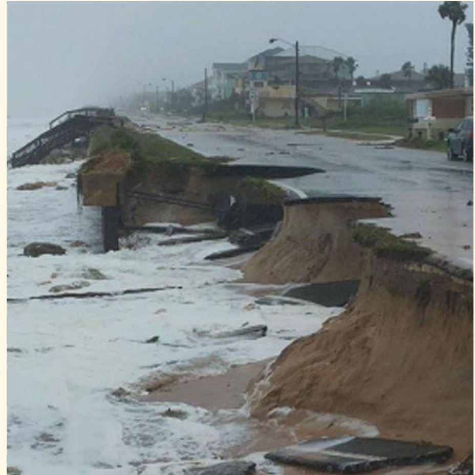
Hurricane Matthew washes away parts of A1A in Flagler County
