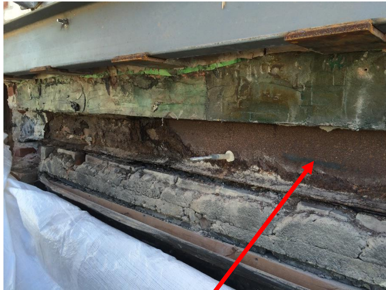
Corroded Steel Beam (note shoring)
