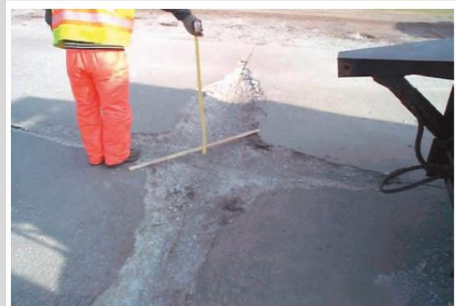
Figure 11-12. V-shaped joints are a common sign of the effects of freeze-thaw damage in concrete pavements. Some joints exhibit an inverted V-shaped deterioration (Courtesy of D. Harrington).
