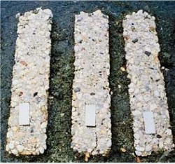
Rating of Concrete: 5 @ 12 yrs Type V Cement W/C = 0.65
