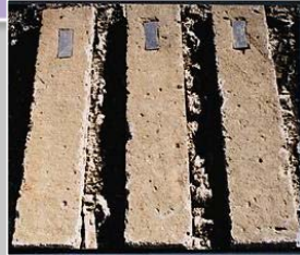
Rating of Concrete: 2 @ 16 yrs Type V Cement W/C = 0.39
